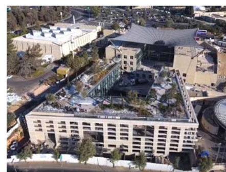
The campus during the construction of the green roof. The tent-shaped roof in the background resembles the temporary tents over archaeological sites and provides for the characteristic appearance of the building.
